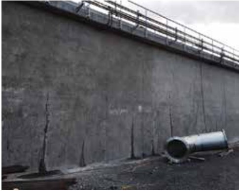
Fig. 3: Vertical wall cracking resulting from base restraint of concrete S&T volume change
