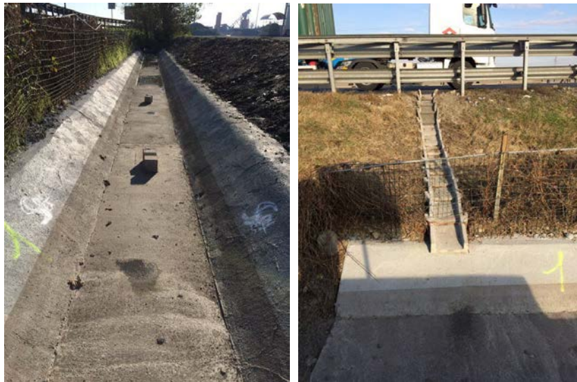
Figure 4 – Culvert (left) and a lateral ditch for water collection from roadway (right)
