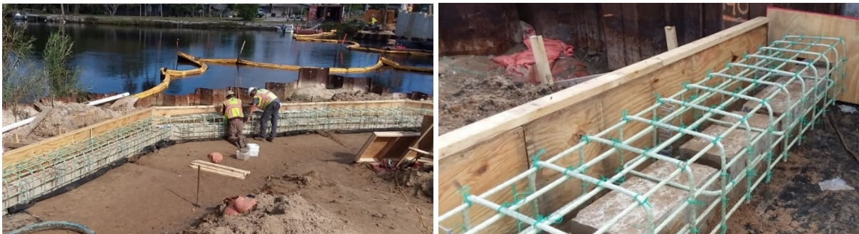
Figure 13 – GFRP bulkhead cap cage
