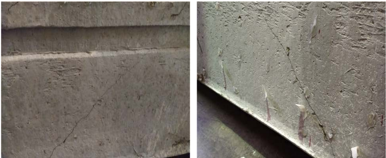
Figure B4 - Test span S1-F1-50-3.5
