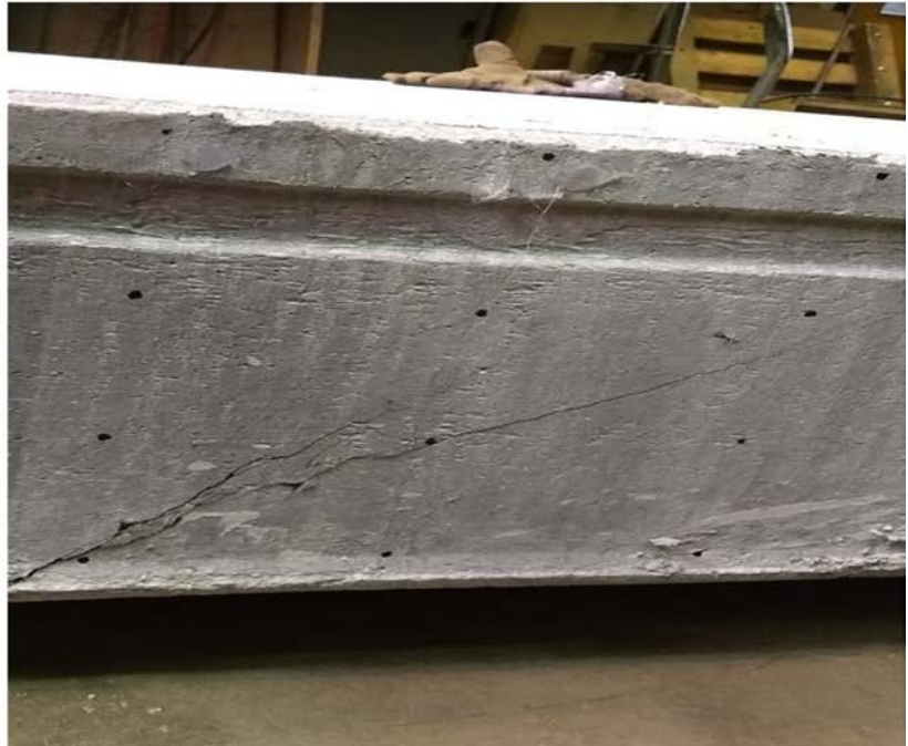
Figure B13 - Test span S1-F2-62-3.0
