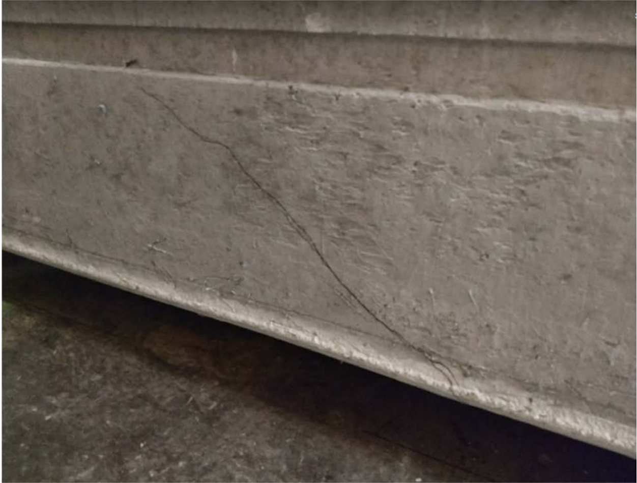
Figure B3 - Test span S1-F1-50-3.0
