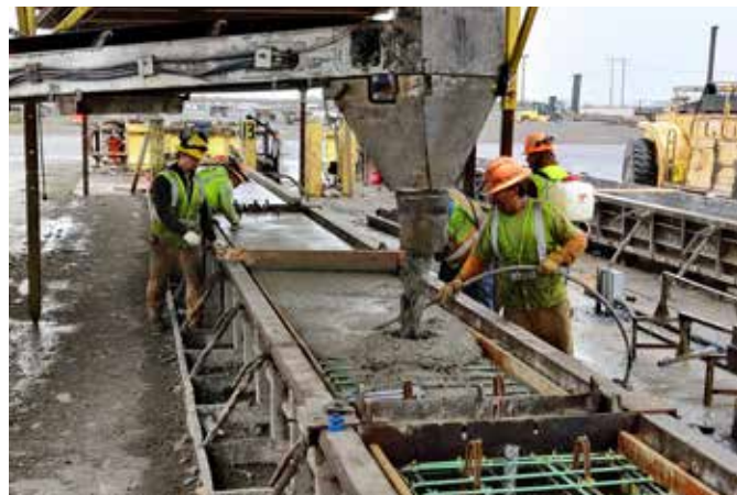
Fig. 3: The 0.1% CNC mixture being placed and vibrated in the prestressed box girder formwork
