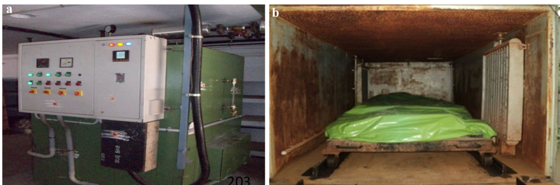
Fig. 3 a Control panel. b Steam chamber.
