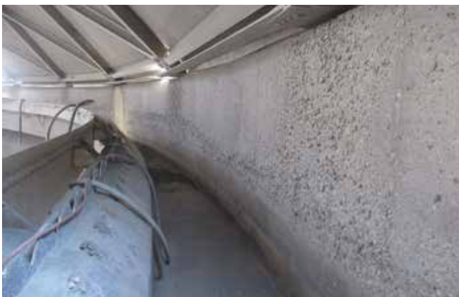
Fig. 1: Concrete surface loss with aggregates exposed due to contact with acids in a water treatment facility (photo courtesy of Wiss, Janney, Elstner Associates, Inc.)
