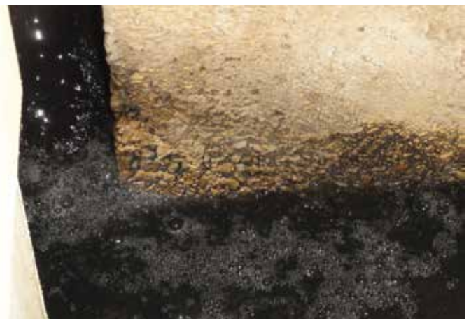
Fig. 2: Concrete damage due to exposure to chemicals (photo courtesy of Wiss, Janney, Elstner Associates, Inc.)
