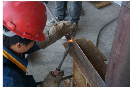
(b) Weld steel bar to the other end of the steel strip
