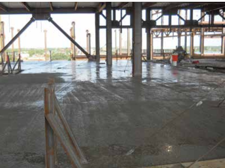
Bleed water coming to the surface prior to finishing (photo courtesy of Arcosa Lightweight)
