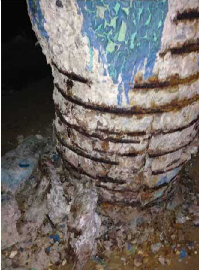
Fig. 2: Spalling that warrants remedial action
