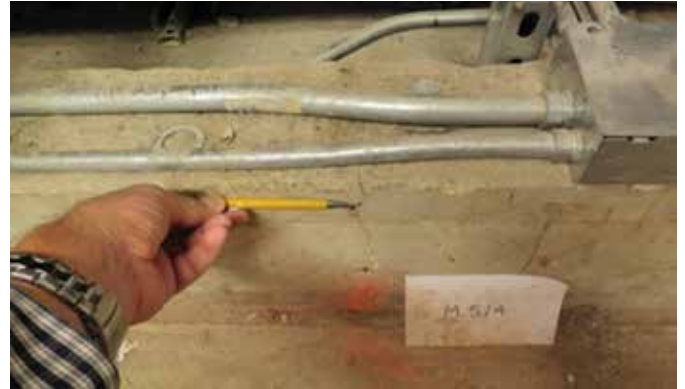
Fig. 3: Concrete cracks, and not all cracks in concrete warrant remedial action
