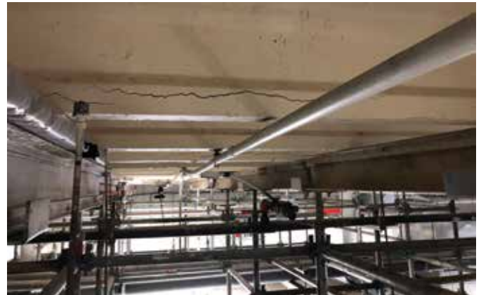
Fig. 4: A crack that warrants remedial action
