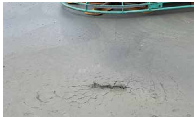
Fig. 2: Surface tearing during troweling
