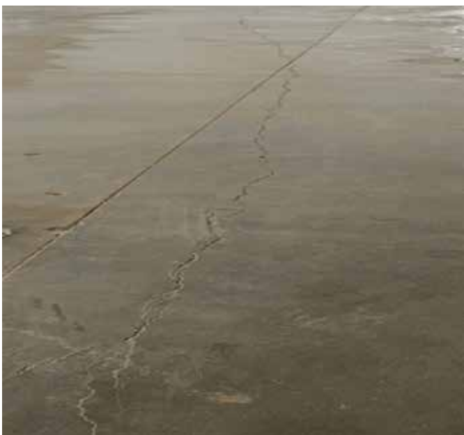
Fig. 10: Saw cutting too late results in cracking (photo courtesy of Scott Metzger, Metzger/McGuire)
