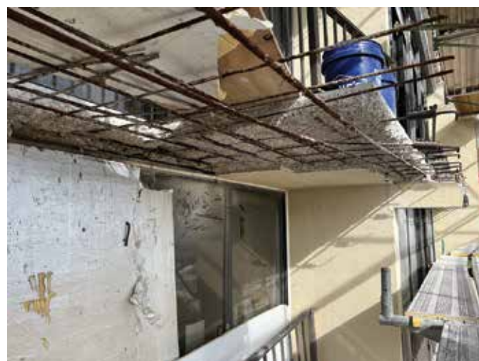
Fig. 5: Corroded reinforcing bars within a balcony (under repair)
