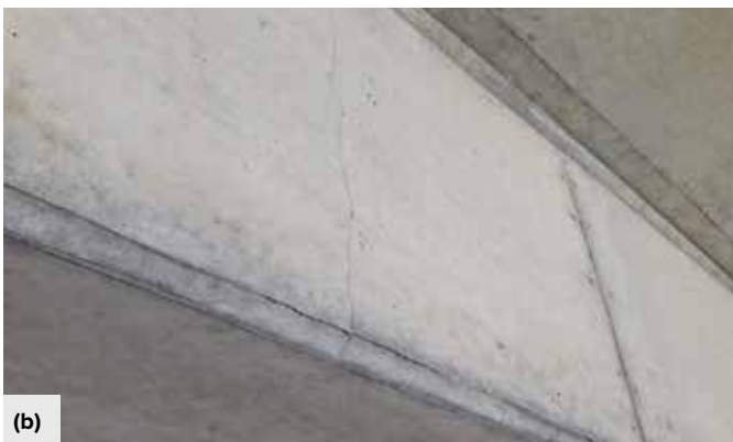
Fig. 2: A beam within a parking garage structure: (a) a general view; and (b) a close-up view of a crack on the beam face and soffit
