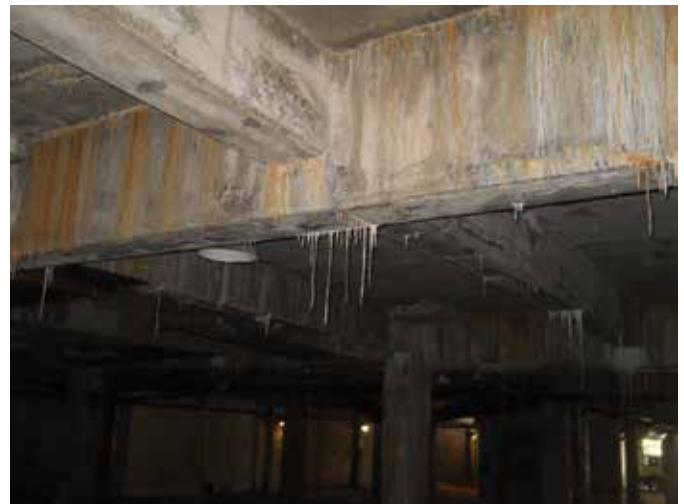
Fig. 1: Leakage with corrosion staining at an existing parking garage framing structure
