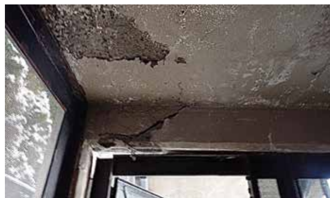
Fig. 4: This wide diagonal crack near a support indicates the need for shoring and additional investigation
