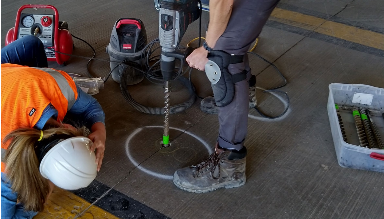
Figure 3-15 Photograph showing the drilling of the chloride penetration sample collection on the ground floor. Current image is of drilling the sample in the wheel-path (according to the paint) and at the epoxy-filled joint.
