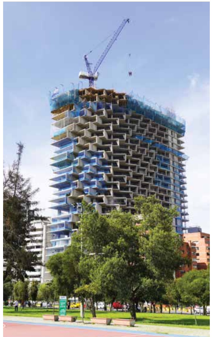
Fig. 6: The construction crane was supported by recently completed floors (photo courtesy of Uribe Schwarzkopf)
