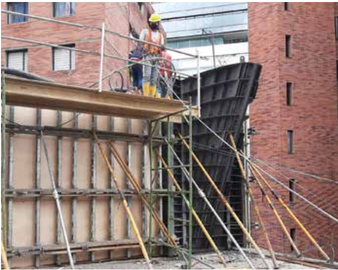
Fig. 7: Steel formwork was reused to build the terrace planters (photo courtesy of Fernando Romo Consultores)
