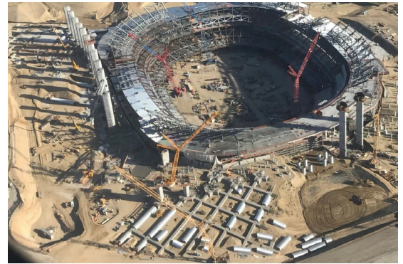
Fig. 3: An aerial view of the construction of SoFi Stadium. The waffle pattern in the foreground is comprised of struts anchoring the blade columns in the soil outside of the MSE fill zone
