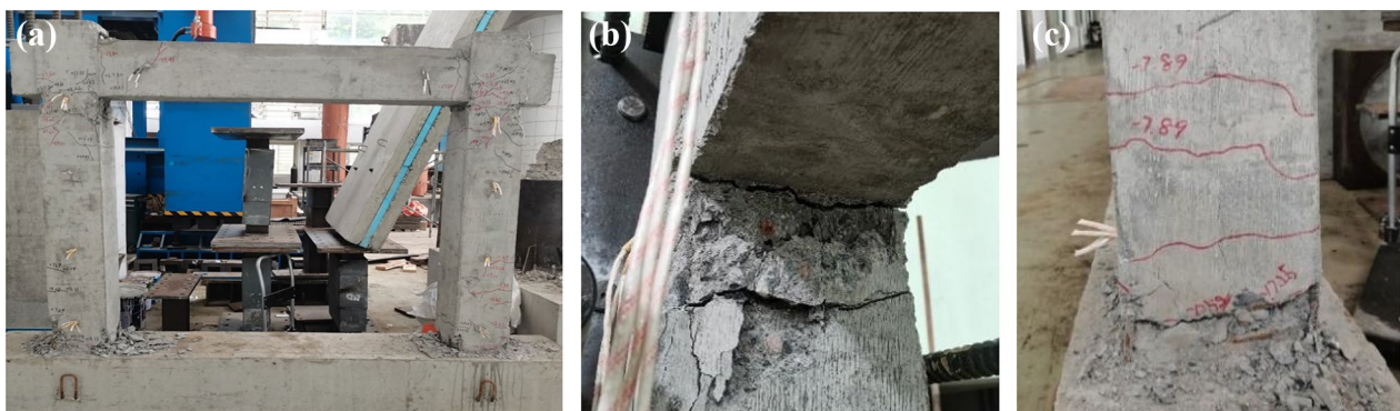
Fig. 13 Detail of the final damage pattern of Specimen 3. a Overall crack development on the front of Specimen 3. b Inner penetration joint of the node. c Damage phenomenon at the bottom of the column
