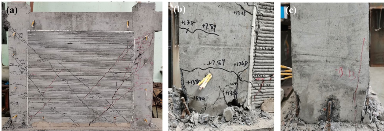
Fig. 11 Detailed drawing of the final damage pattern of Specimen 1. a Overall crack development on the front side of the specimen. b Left column bottom damage phenomenon. c Right column bottom damage phenomenon
