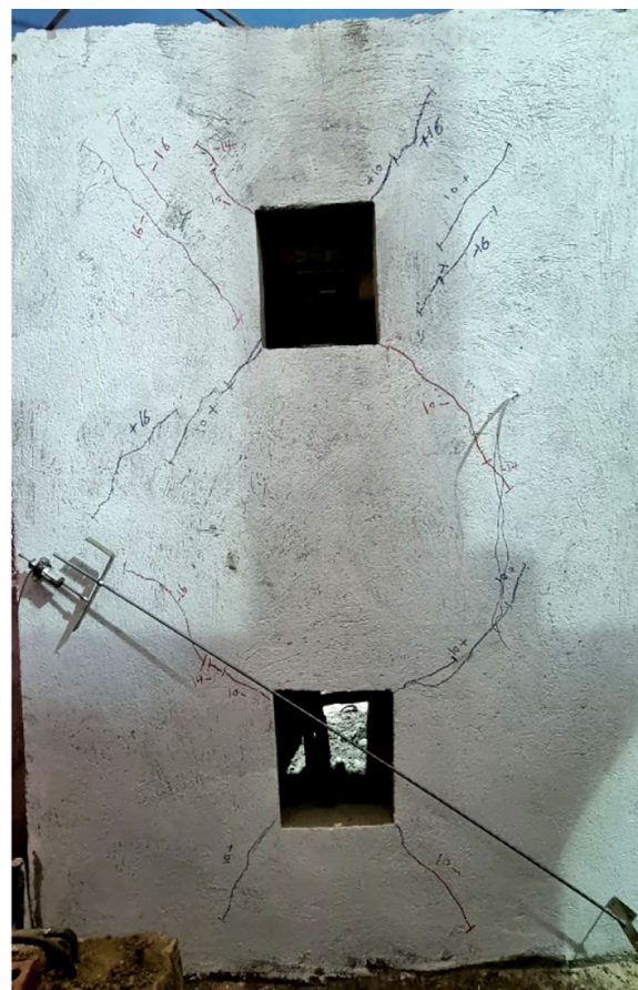
Fig. 16 The first obvious cracks S-02 (back)
