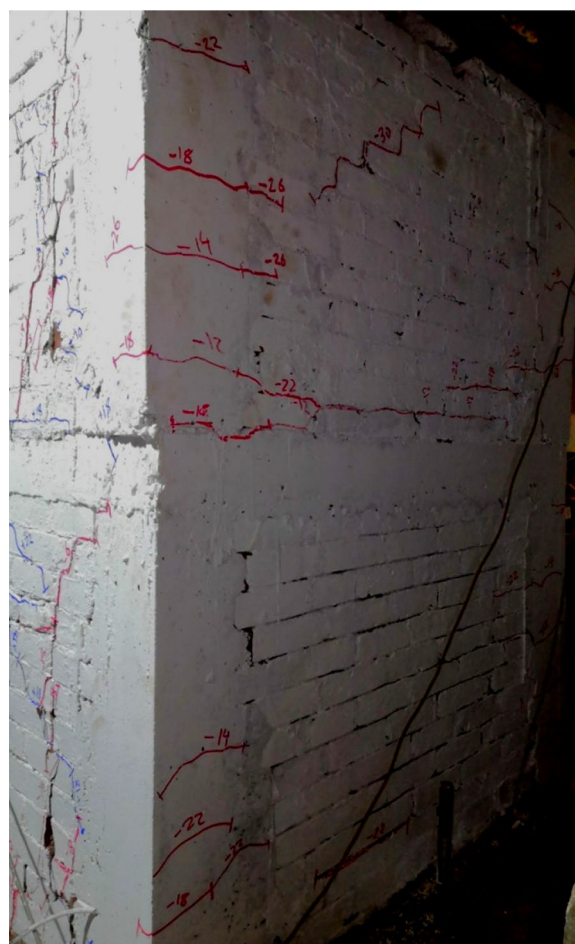
Fig. 14 Crack failure pattern S-01 (front)
