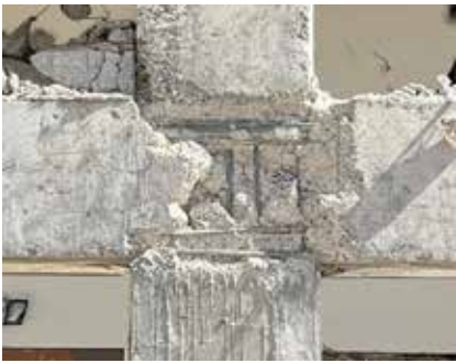
Fig. 6: Beam-column joint with unconfined beam reinforcement, Turkey, 2023
