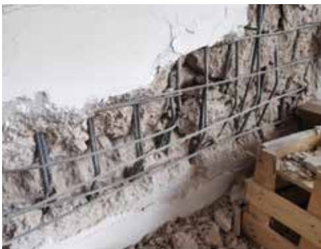
Fig. 3: Failure of wall with light lap-spliced vertical reinforcement and no boundary-element confinement, Turkey, 2023
