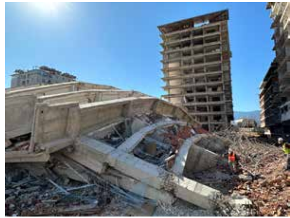
Fig. 7: Building that overturned with “better” reinforcement details (foreground), and a building with 6% residual drift ratio (background), Turkey, 2023
