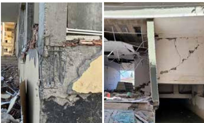
Fig. 4: Failure of column (left) and structural wall (right) without adequate confinement within the foundation near an edge, Turkey, 2023
