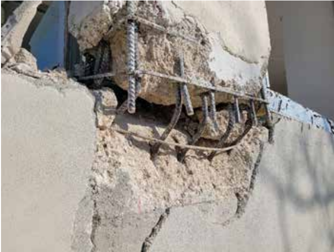
Fig. 5: Failure of a column without adequate confinement within the foundation near an edge and lap spliced bars immediately above the foundation, Turkey, 2023
