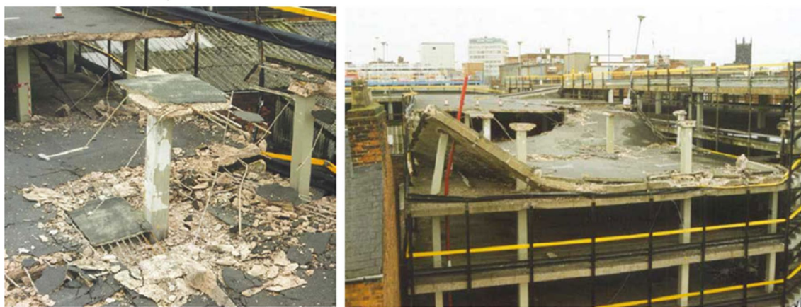
Fig. 1 Punching shear failure at slab–column connections: Piper’s Row Car Park, Wolverhampton, UK, 1997 (Wood, 2003)
