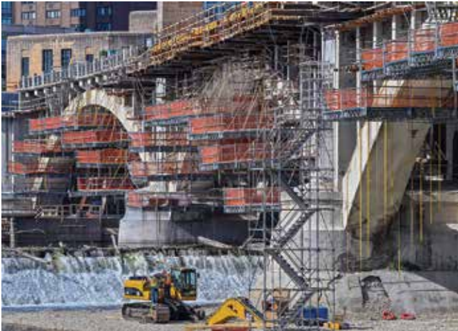
Access to the substructure required complicated suspended scaffolding and dewatered cofferdams (photo courtesy of Joe Szurszewski Photography)
