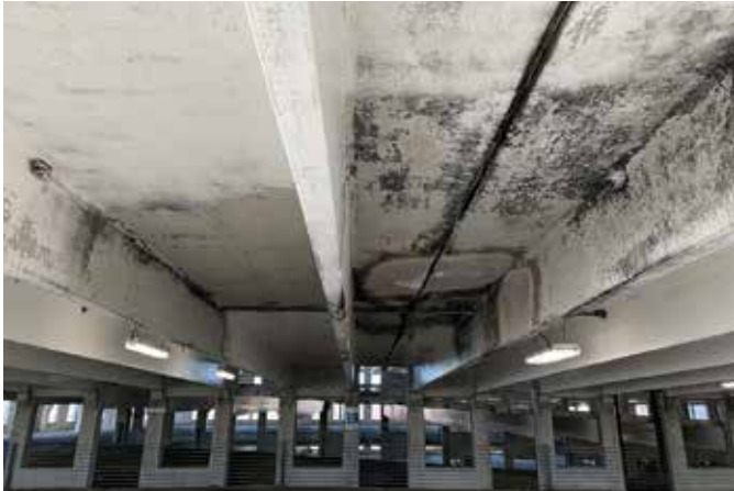
Fire damage to the underside of the level four precast double tees
