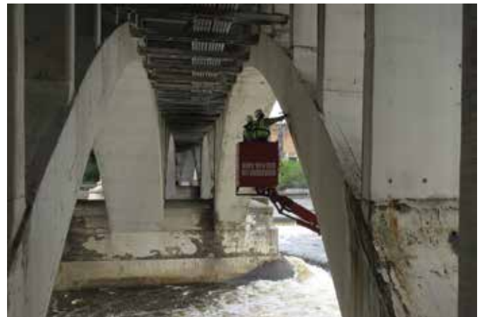
Hands-on inspection from under-bridge inspection unit, showing deterioration of arch ribs and pier bases
