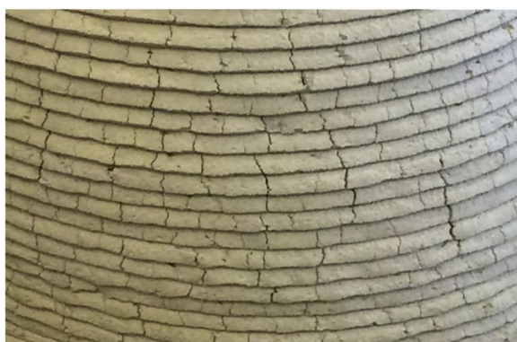
Fig. 1 Excessive shrinkage cracking of 3D-printed sample (Schutter et al., 2018)
