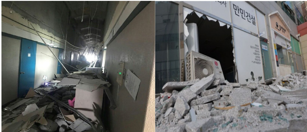
Fig. 3 Example of earthquake damage. Source: Architectural Institute of Korea (AIK), damage to non-structural materials described in the Pohang earthquake report, https://www.aik.or.kr/html/page05_05.jsp
